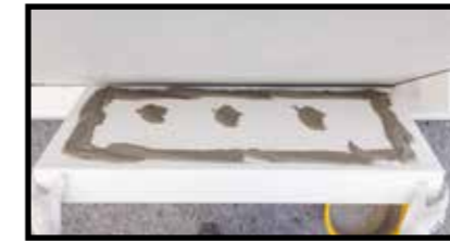
Installation of isolating panels with a notched trowel in a vertical direction
